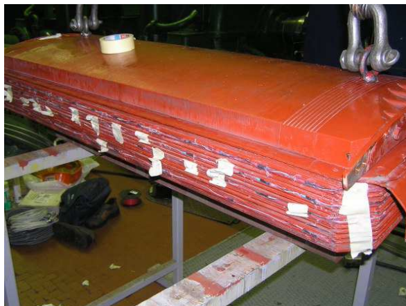
Fig 6. Photo of pole winding in HPP Vinodol during the process of temperature sensor installation.
